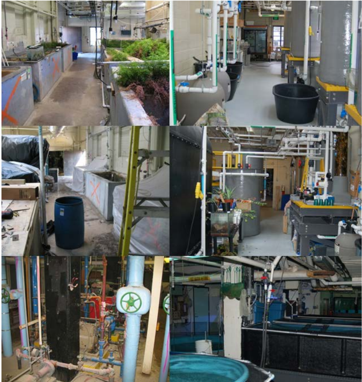
Figure 1: Three before-and-after sets of photos of service areas. Photos on left were taken 2009, photos on right taken from same vantage points in 2012. Top: freshwater wing showing concrete reserve tanks (left) and open-system tanks; after construction (right) note epoxy sealed floors and walls and LSS equipment. Middle: a section of the marine wing before and after; the back wall in both pictures denotes the line of 1936/1963 construction. Bottom: the aquarium's basement, showing the remnants of the chilled water system (left) described by Moore (1965), this was one of the first large-scale chillers ever used in a public aquarium. The area was converted to a modest quarantine area (right).
