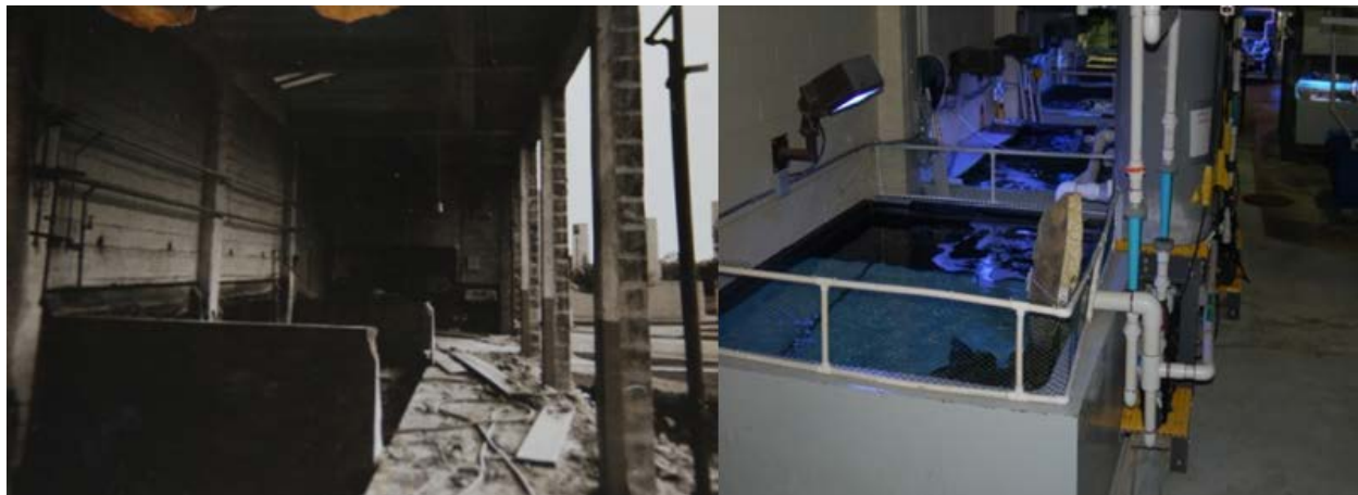
Figure 3: The concrete tanks that had limestone and bleached coral inserts to create reef habitats as described by Moore (1965). Photo at left shows the tanks (and the marine wing itself) under construction in 1963, photo at right shows the same tanks in operation today. Photo on the right by Jeff W. Moore.
